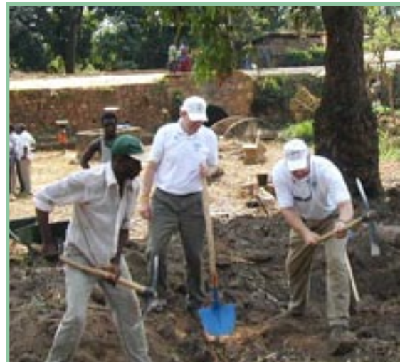
Togolese and U.S. Rotarians dig a trench as part of a project to supply clean water to residents of Midoudou, Togo.
